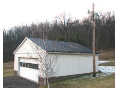
ENCROACHMENT ISSUE: A minimum of 20 feet of clearance on each side is required around power lines and equipment.
