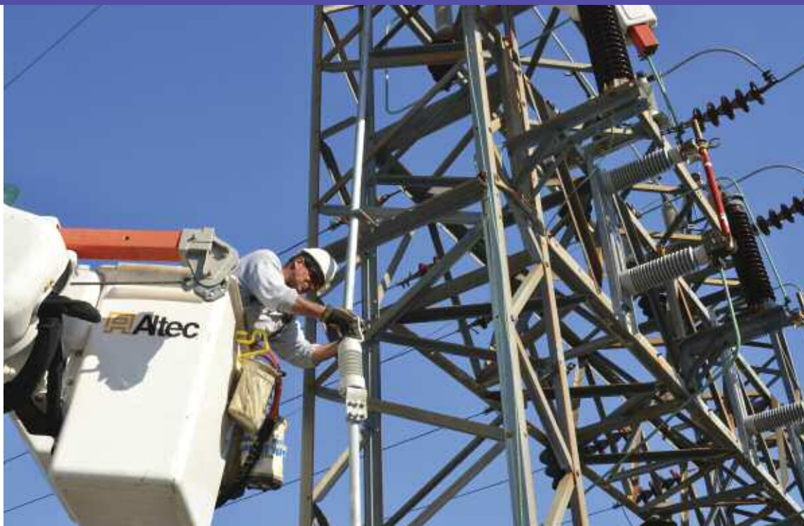
AT LEFT: Martinsburg District Crew Leader Greg Dilling installs an in-line insulator in piping at the Frankstown Substation. The pipe is part of a new switch assembly installed during an improvement project.
