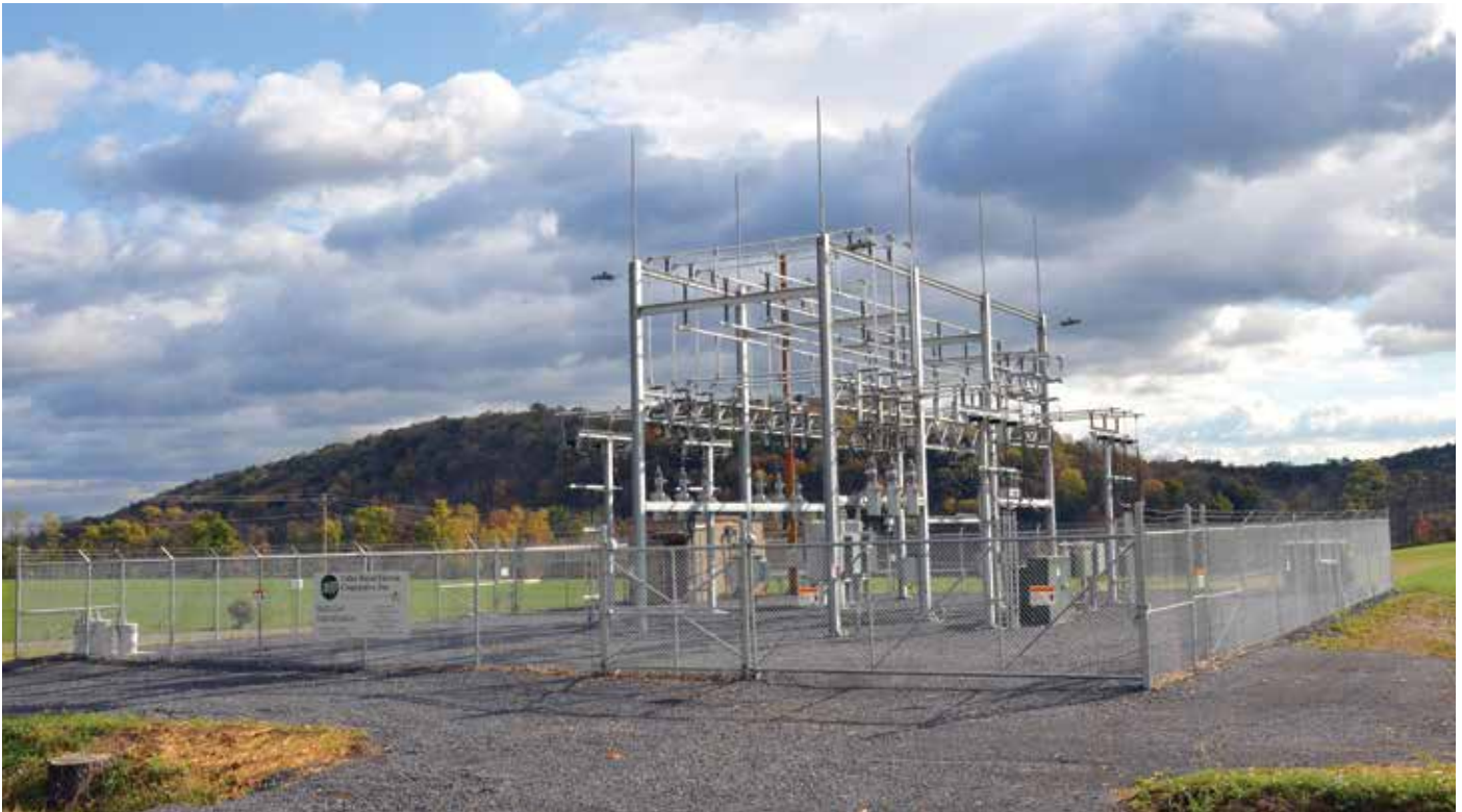
ABOVE: Valley REC's new Reeds Gap Substation is located along Route 35 in Juniata County. It replaces a substation that had been in service since the early 1950s. Below: The construction project also includes some pole replacements in the vicinity. Photos by Doug Roles
