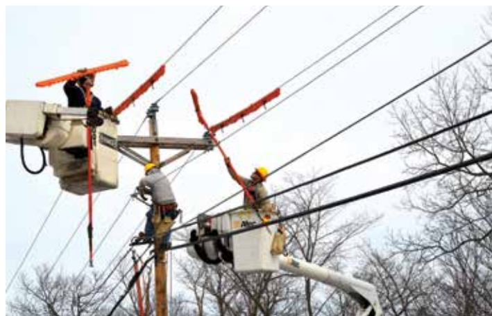
WORKING TOGETHER: From left, Journeyman Linemen Adam Atherton, Justin Berrier and John Fogelsonger move an energized line in preparation for setting a new pole.
