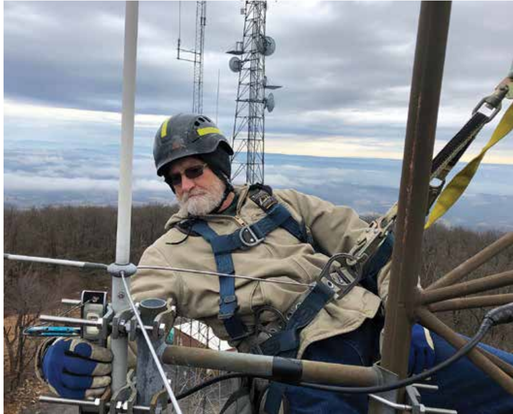
FROM THE TOWER: Jerry Cox, of MultiComm, Inc., hangs from the co-op’s Loop Mountain tower performing some maintenance work on the antenna used to serve the local amateur radio community in Huntingdon County.
