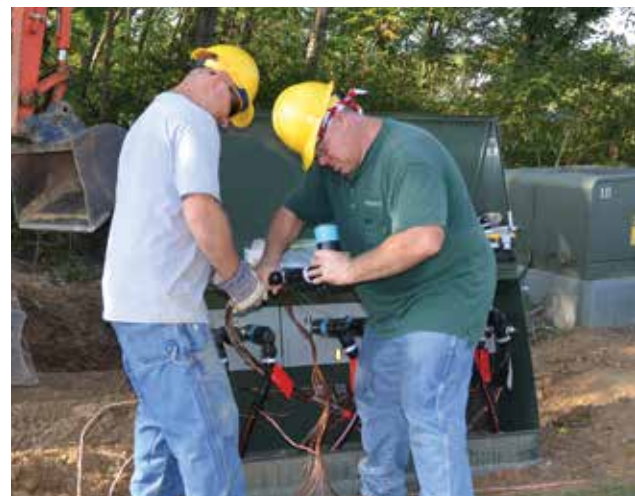
RIGHT: Staking Engineer Jason Hey, left, and Journeyman Lineman Bill Bogel install an elbow on a new piece of underground line.
