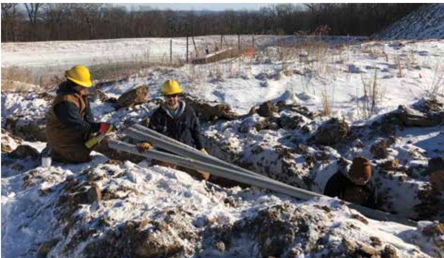
NEW CONDUIT: From left, Martinsburg linemen Ryan Dodson and Trevor Eichelberger work with electrician Zach Yohn as they lay conduit for an underground service at Blue Knob Ski Resort.
