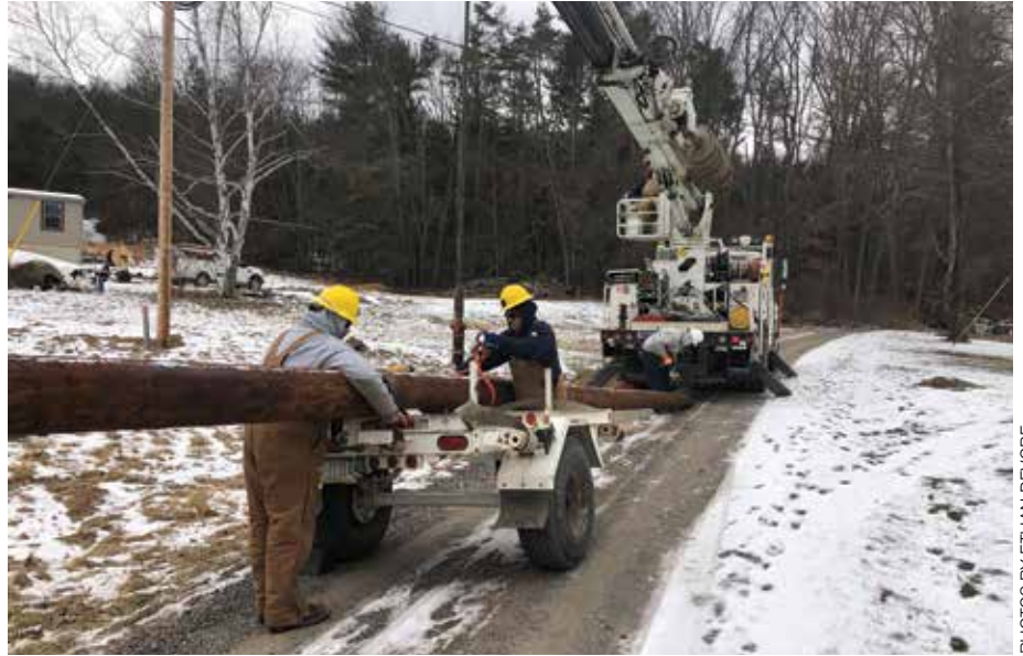
LINEMEN AT WORK: Huntingdon linemen Matt Fagan, left, Curt White, middle, and Justin Berrier, right, work with equipment operator Rich Sunderland, top, as they prepare to set a new pole on Valley REC lines.
