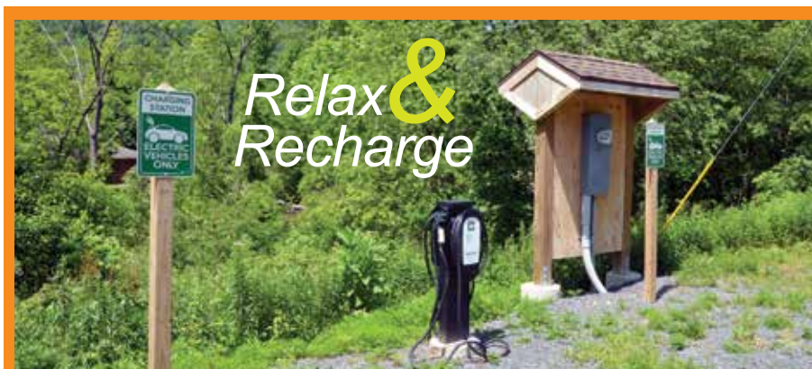
Visitors to Greenwood Furnace State Park, Huntingdon County, can charge their electric vehicles at this station while enjoying the park. A charging station is also available at Cowans Gap State Park, Fulton County. In the fall of 2018, the Pennsylvania Department of Conservation and Natural Resources began an initiative to place EV-charging stations at 40 state park locations. Twenty-three have been installed to date. PHOTO BY DOUG ROLES
