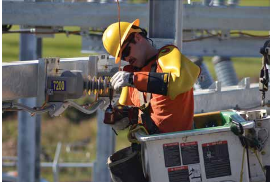
ABOVE: Working from a bucket, Fourth-Class Lineman Josh Gutshall installs wiring for substation metering equipment.
