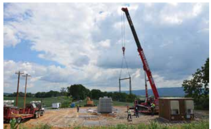
ENERGIZED: A crew from Bryce Saylor & Sons, Inc. Crane & Rigging Service places a substation transformer and a substation control building at the new Sinking Valley substation in Blair County in early August. Valley REC employees and crews from Tri M Group, LLC and Hickes Associates, Inc. were on-site to assist. This new substation will be closer to a Penelec 46-kilovolt supply line, reducing the likelihood of a service interruption. Construction should be complete about the time this issue of Penn Lines arrives in mailboxes.
