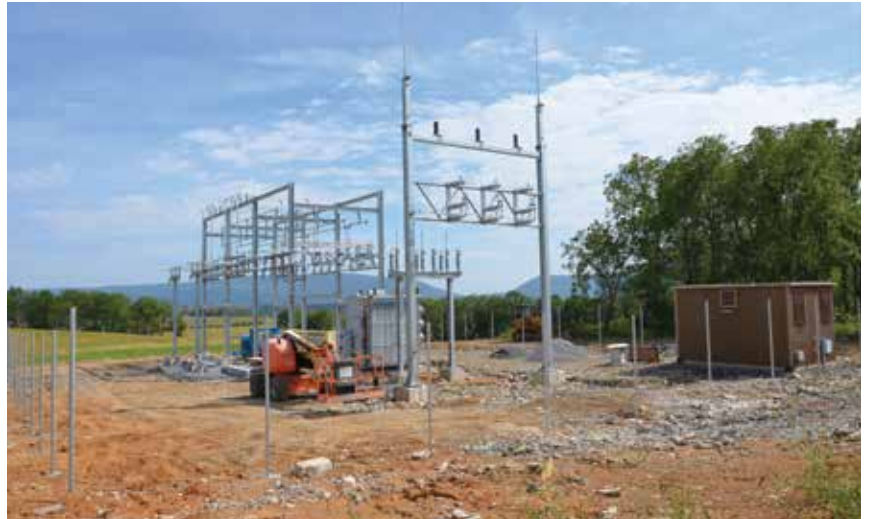
FINAL STRETCH: Construction of Valley REC’s new Sinking Valley substation is nearly complete. In this photo from late September, poles have been erected for fencing.
