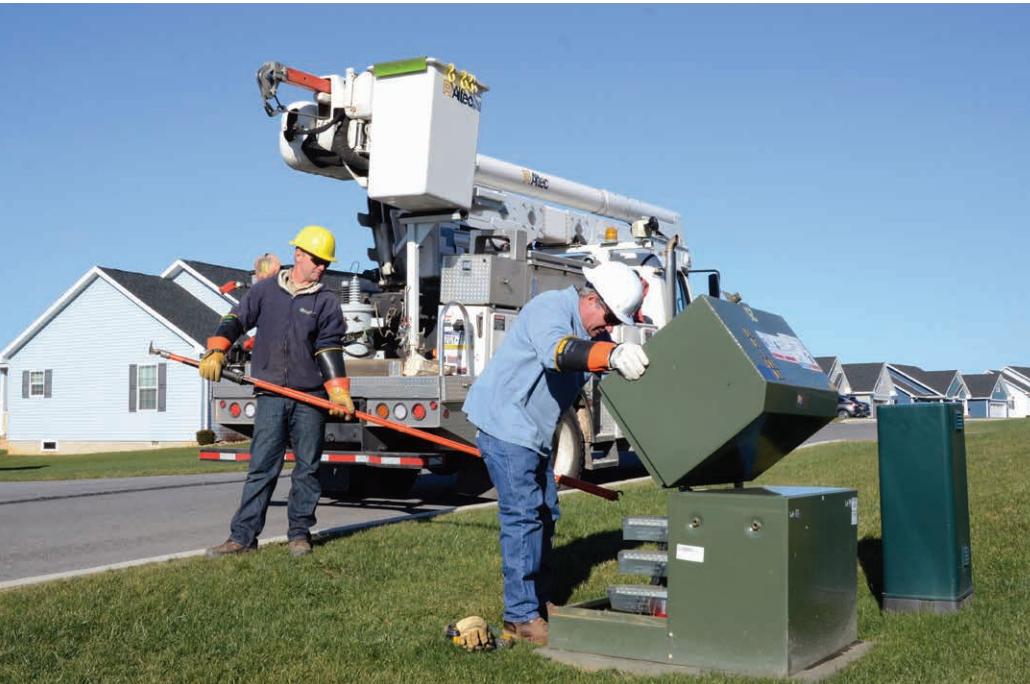
GOOD LOOKS: Valley Rural Electric Cooperative Crew Leader Greg Dilling, right, and Journeyman Lineman Ryan Dodson inspect a pad-mounted transformer at the Graystone Cottage Community.
