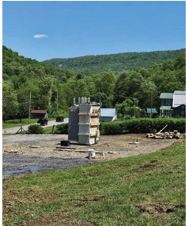
NOT MUCH LEFT: By mid-May, the only thing left of the original Three Springs facility was the substation transformer. In early June, crews used a crane and truck to move that piece of equipment to the Clear Ridge substation.
