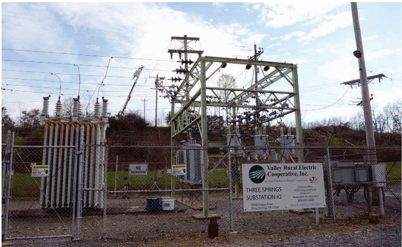
END OF AN ERA: Valley Rural Electric Cooperative crews will begin replacing the Three Springs substation, built in the 1950s, with a new facility on the same site in Huntingdon County. Associated lines are also being converted from 14,400 volts to 25,000 volts to increase service quality and reliability.
