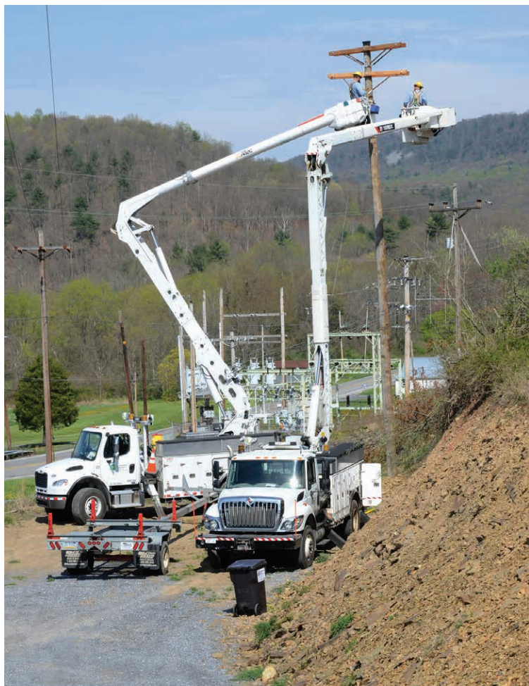
GETTING STARTED: Valley Rural Electric Cooperative crews set a new pole near the Three Springs substation on April 17. Several poles were erected near the substation to enable rerouting of power from another co-op substation to the nearby Southern Huntingdon County High School.
