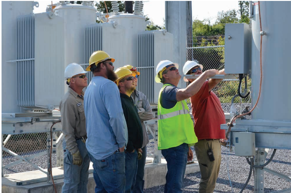
COMMUNICATIONS CHECK: Valley REC Vice President of Operations Todd Ross, second from right, and Coordination Engineer Eric Henchey, right, ensure substation communications equipment is working properly. Also shown, from left, are: Crew Leader Tink Bucher, Journeyman Linemen Logan Booher and Curtis Starr, and Second-year Lineman Nathan Berry.
