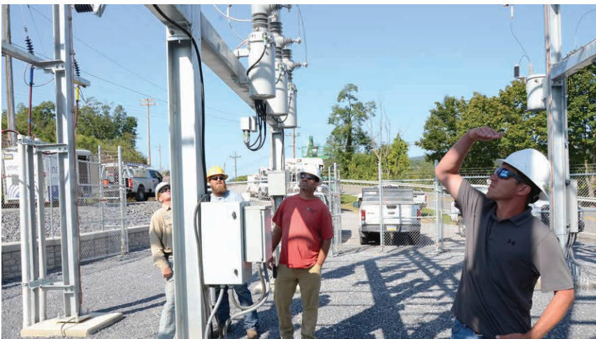
LOOKS GOOD: Shade Gap District Manager Brandon Clemens, right, inspects equipment in the new Three Springs substation. In the background, from left, are: Crew Leader Tink Bucher, Journeyman Lineman Logan Booher and Coordination Engineer Eric Henchey.
