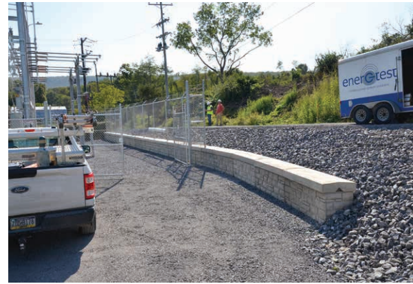
CONCRETE FEATURE: Big Valley Concrete, a Valley REC member, cast and stamped this retaining wall, which was set in place by another co-op member, Scott Bishop of Bishop's Loggin-N-Haulin.
