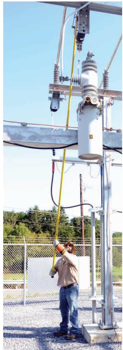
POWERING UP: First-year Lineman Matt Fish closes a bypass switch as crews energize the Three Springs substation on Sept. 5.
